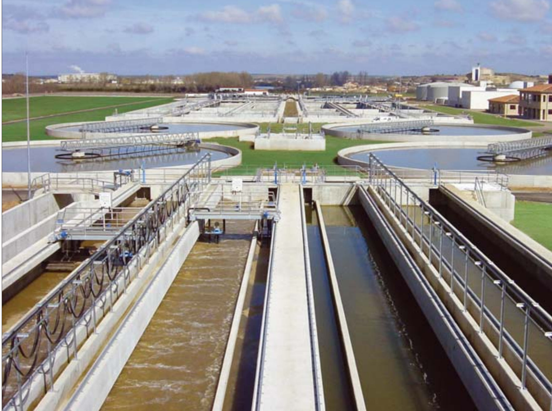
Wastewater treatment plant in Salamanca.
